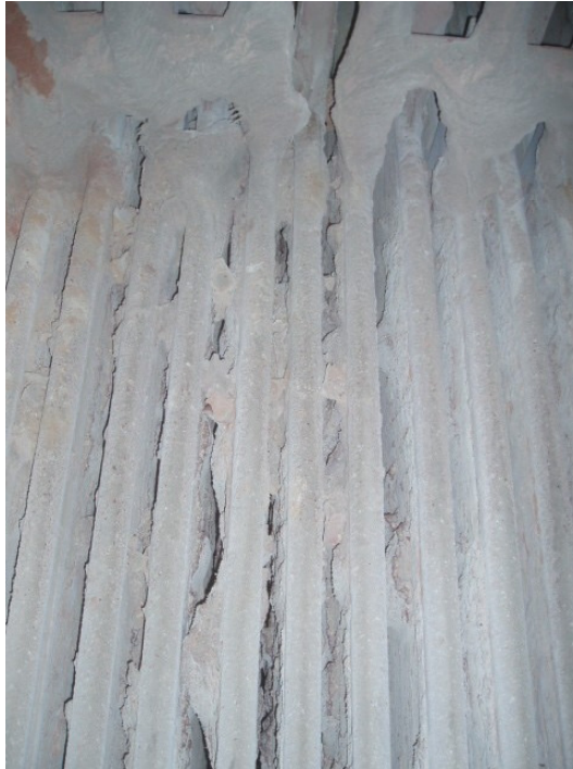
Fouled upper bank LTSH
